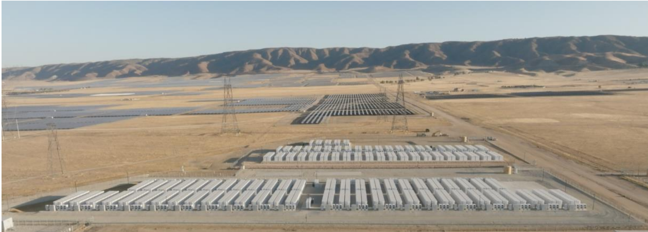
Representative BESS yard for illustrative purposes of defensible space. Not Rancho Viejo visualization
